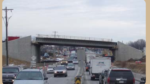
The Parkway will cross over Route 309. The structure features a cobblestone look and the Montgomery Township logo.
