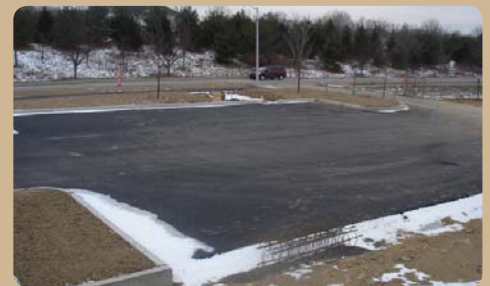
The addition of the Knapp Road trailhead parking lot will give users free parking and easy access to the Shared Use Path.
