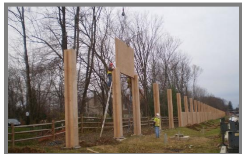
Photo 1: Workers prepare to set panels for a noise wall along DeKalb Pike
